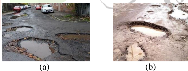
Fig. 1: Road Damage causing potholes and craters
