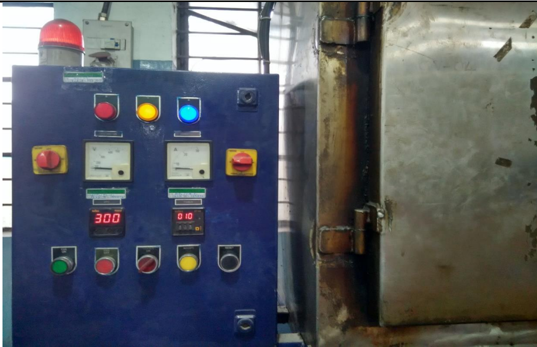
Figure 4. Control Panel of furnace
