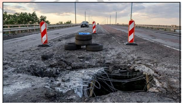
Figure 3.1. damage bridge deck
