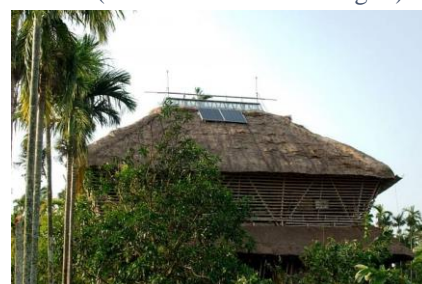
Figure 3.5 Solar panels at the roof (Source: downtoearth.org.in)
