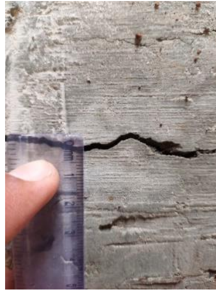
fig. 8 Crack found on column
