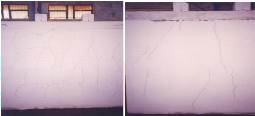
Plate 4. Typical crack pattern of wall after encasement.
