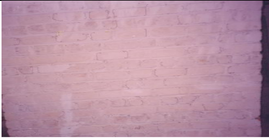
Plate 3. Typical crack pattern of Walls before encasing.
