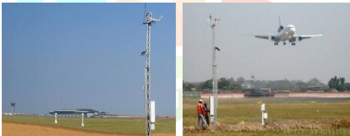
Fig. 5.1 Wind speed and Direction sensor installation at Airport
