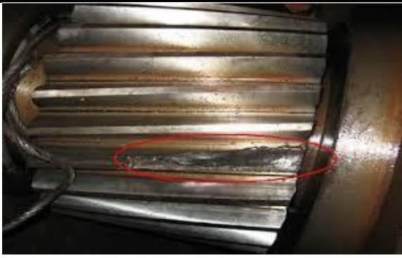
Fig .3.1 Damaged Helical Gear of Gearbox
