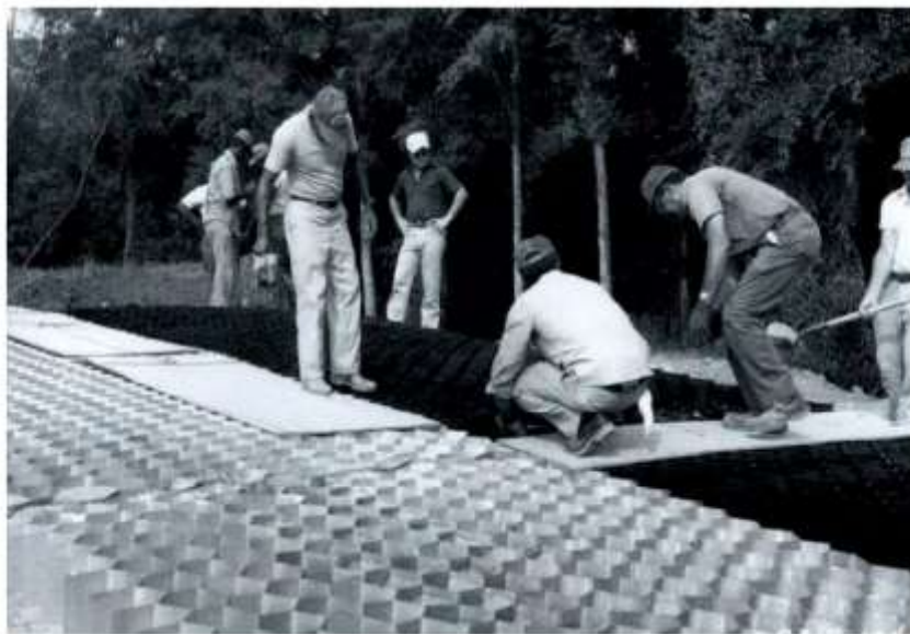
Figure 3.1 Early version of Geocells used by US Waterways, Experimentation Station at Vicksburg, MS, USA
