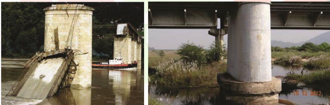
Figure 2.1 Collapsed and eroded bridges due to sand mining
