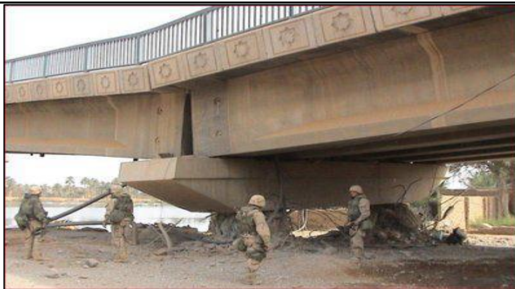
Figure1.1.A bridge in Iraq damaged by a relatively small amount of explosives placed in a terrorist attack [3] .
