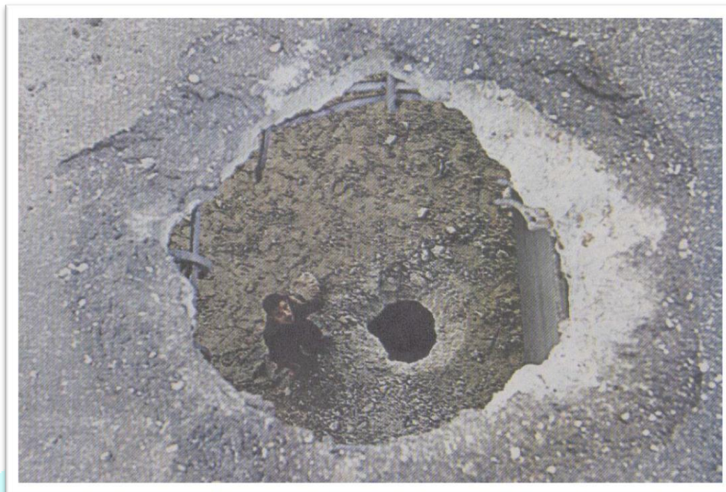
Figure.1.5. Damage to a Bridge in Palestine after a Missile Attack [3] .
