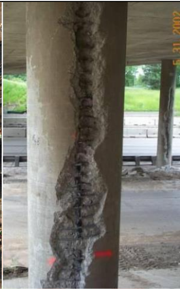
Figure 1.8. Column Damage due to explosion under bridge
