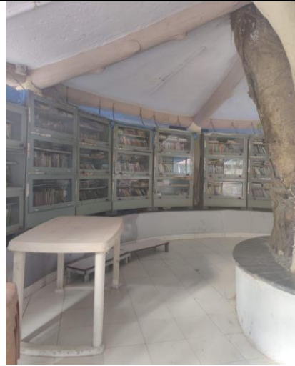
Image 17 -Inadequate space, lighting & ventilation in Library space
