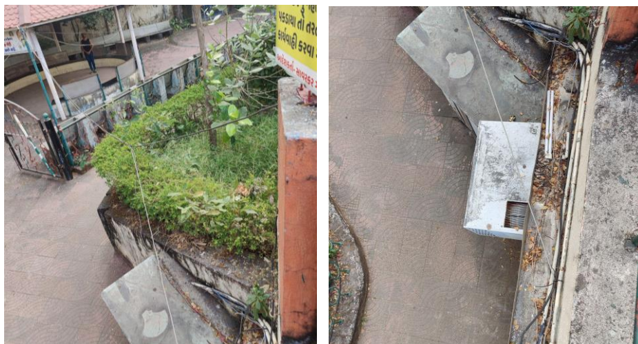
Image 15 (left) & 16 (right) - Inadequate artificial lighting & non-maintained installation
