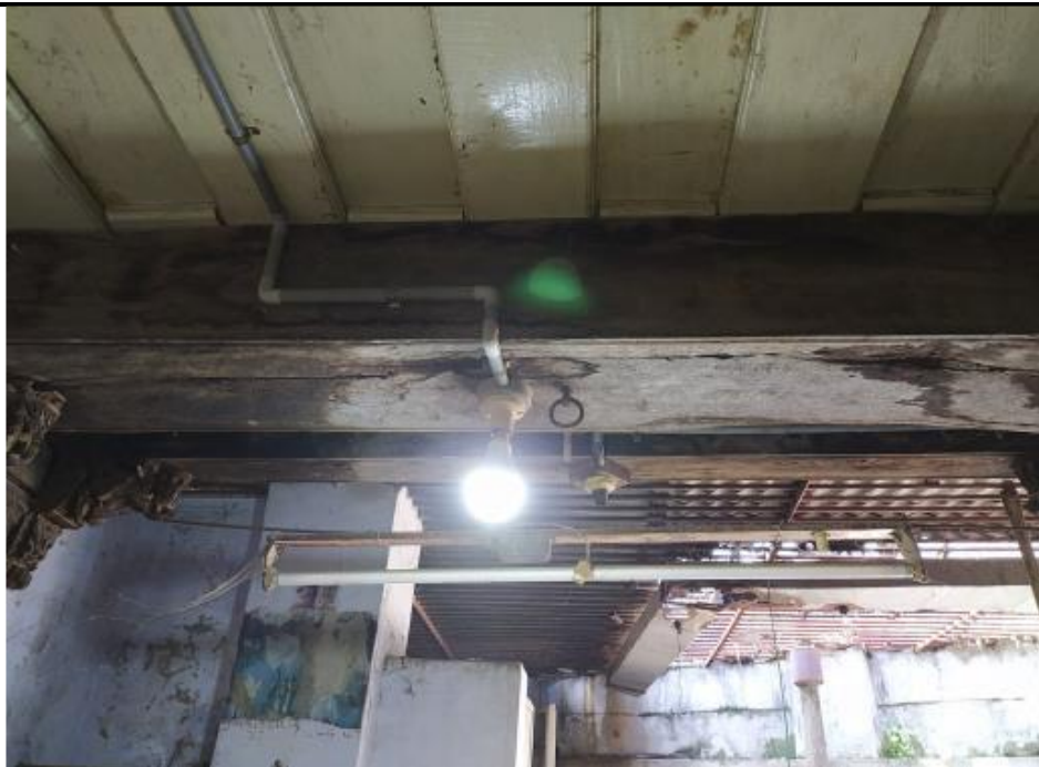
Fig 36 Entrance weaker portion
