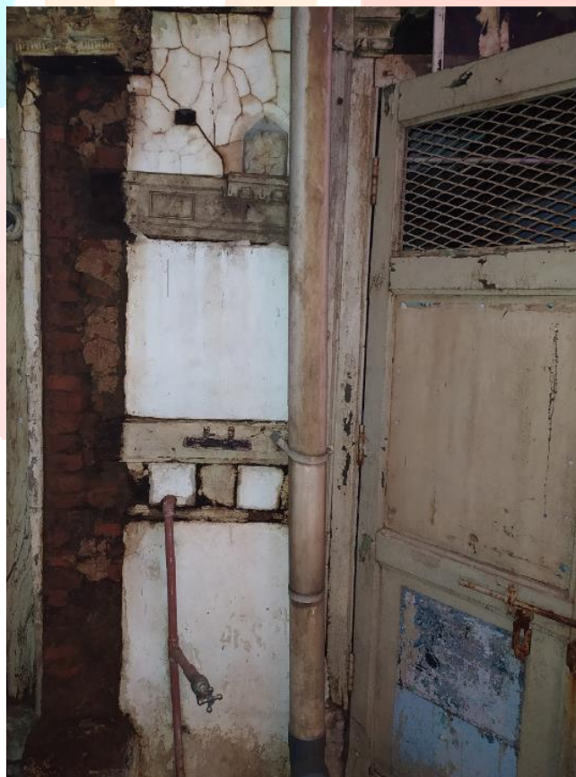
Fig 39 Failed bathroom column
