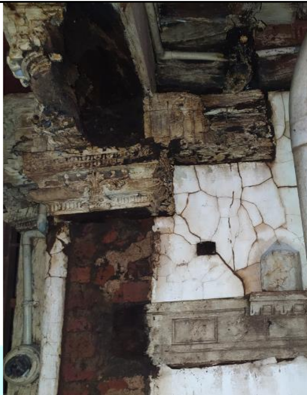
Fig 38 Failed bathroom column
