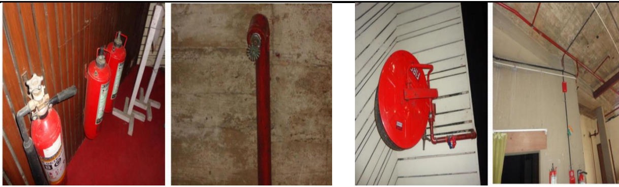
FIGURE 13: Fire safety Device
