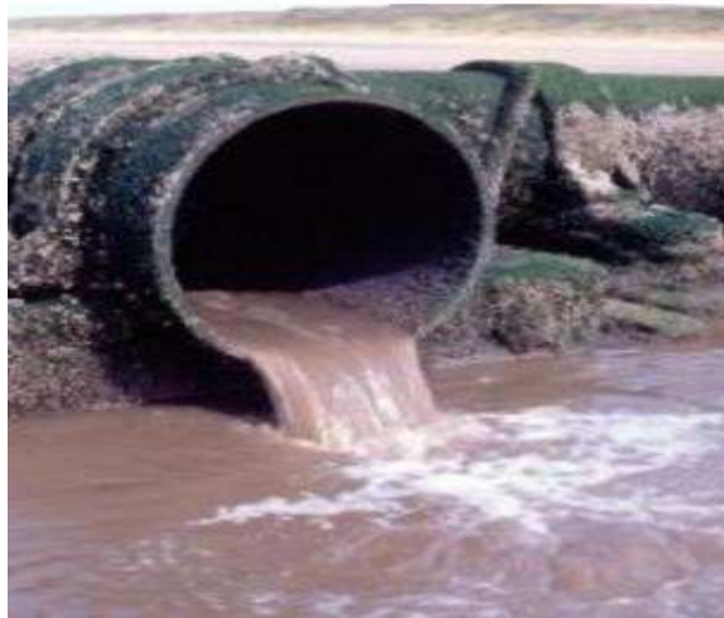
Figure 1.1. Discharge of Untreated Industrial Waste Water
