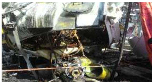
Fig 1- Catastrophic view of transformer after burst and fire.
