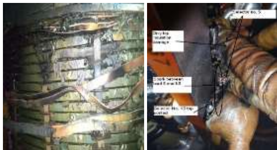
Fig 2 & 3 – Winding deformation & insulation failure.
