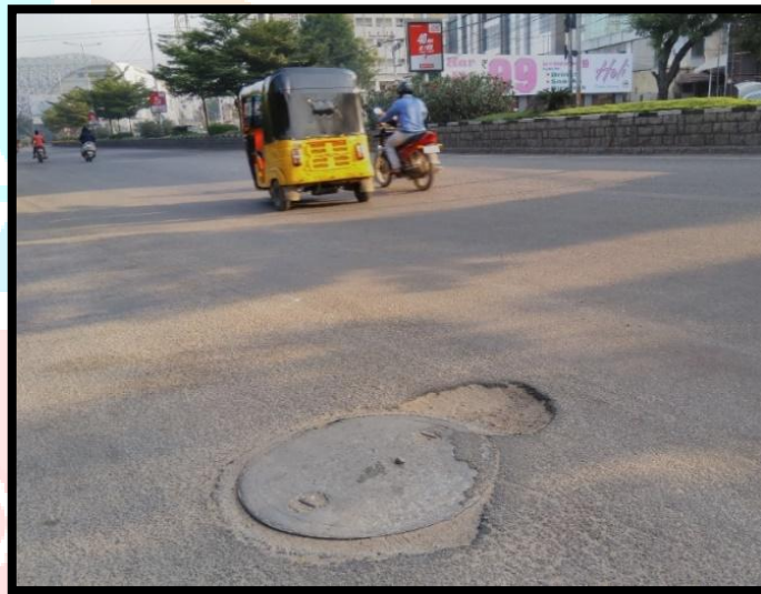
Fig 7: Potholes at usual repair point like manholes
