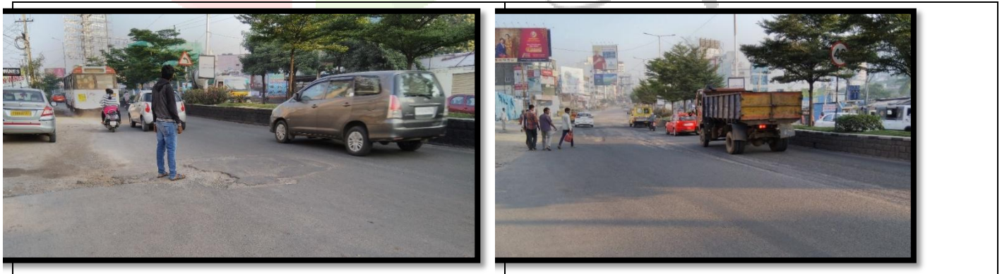
Fig 3: The road totally damaged and raising the dust when heavy vehicles move on it
