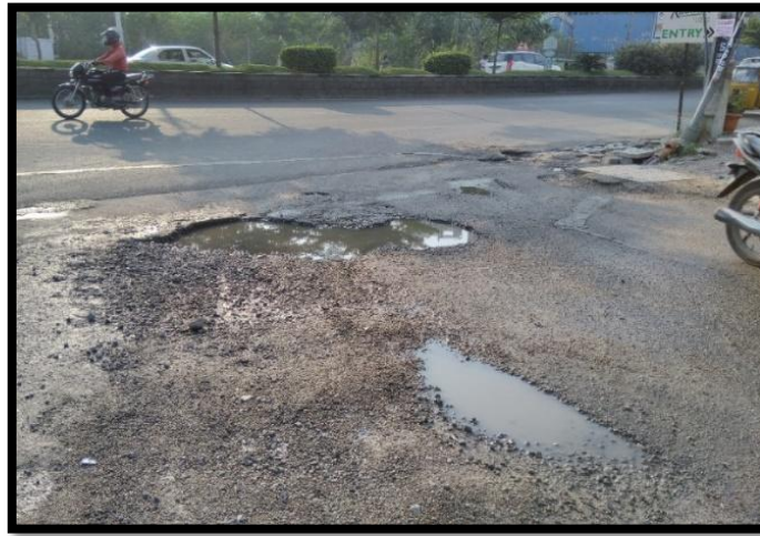
Fig 6: Potholes at water logging areas
