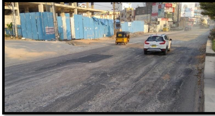
Fig 4: Patch work has done on the potholes, but this cannot be useful for the long life
