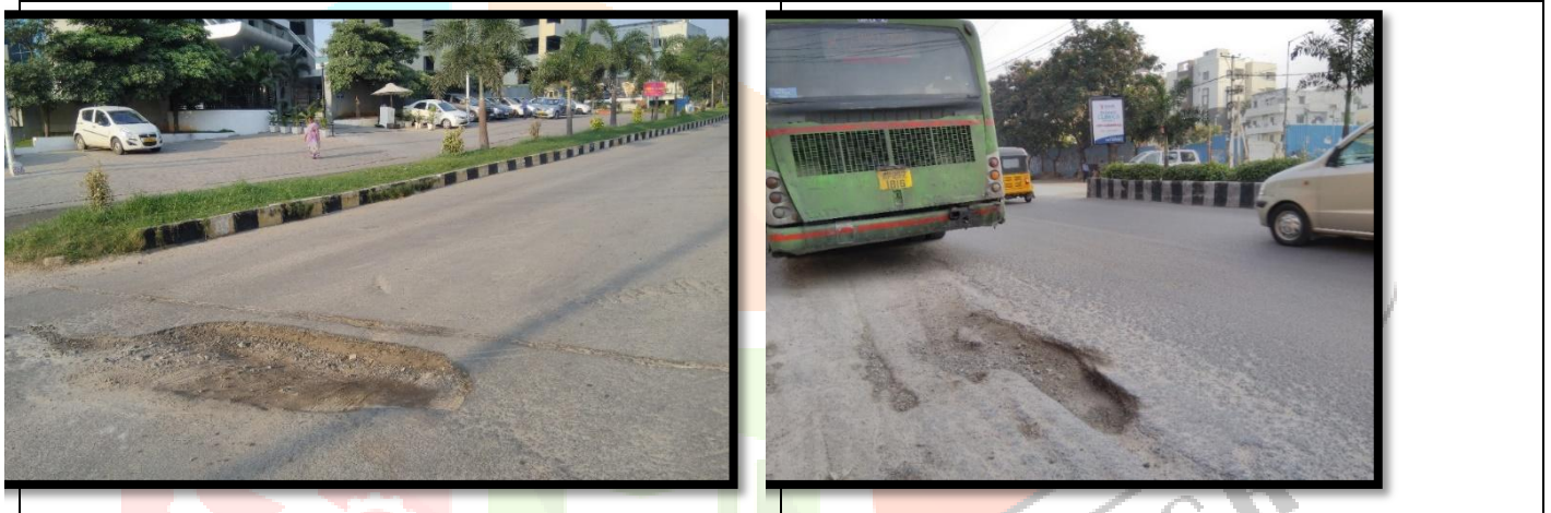
Fig 5: Deep pothole on the center of the road is a great hazard to the vehicular
