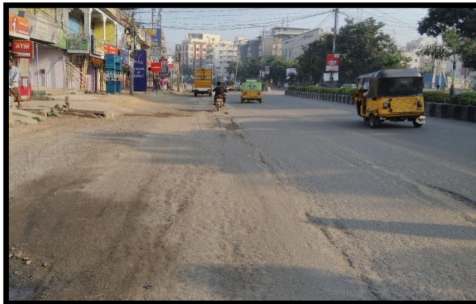
Fig 8: Potholes occurring at the bus stops causes a serious hazard to the passengers
