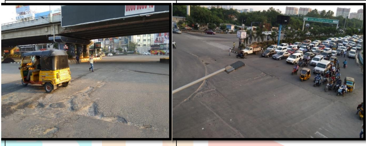
Fig 2: Potholes at the intersection causes traffic congestion
