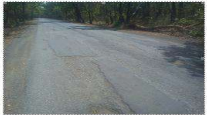
Figure 2 Rough road condition
