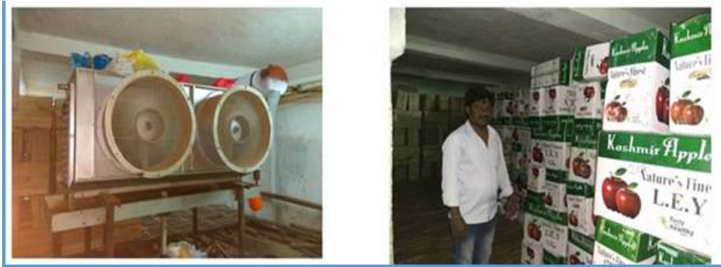
Fruits and Vegetables Storage rooms with Cooling System
