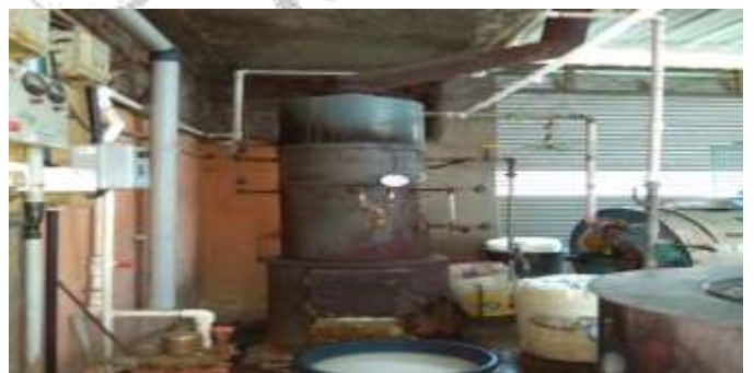
Fig 1.2 steam boiler for heating of clothes
