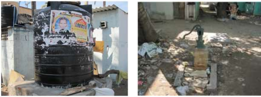
Fig 14. Water supply through tanks and stand pipes.
