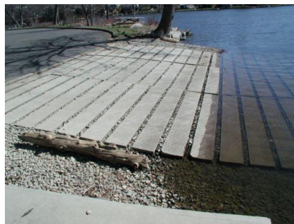
Figure-27- Anti skid Ramp
