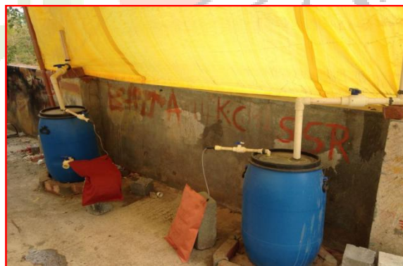
Fig.4: Digestion tank with air pillows.
