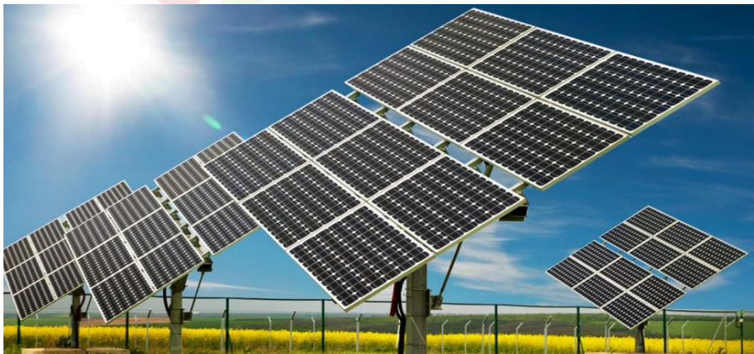
Fig 3.2 Solar panel arrangement
