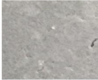
Figure 5. Image with No Surface Crack
