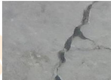
Figure 6. Image with Surface Crack
