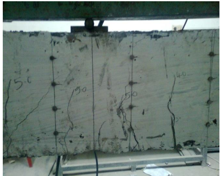
Fig. 2 Showing shear cracks
