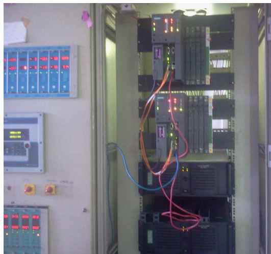
Fig. 3. Actual view of both the controllers, Above two are New Programmed PLC and Below two are DCS.
