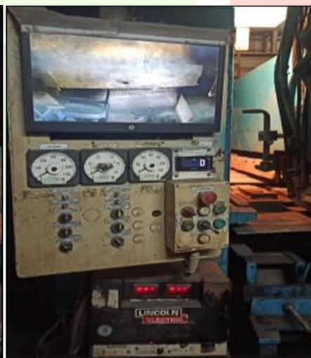
Fig. 9 Control panel with camera setup
