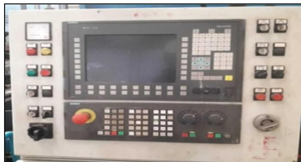
Fig. 3 Control panel of SCCM
