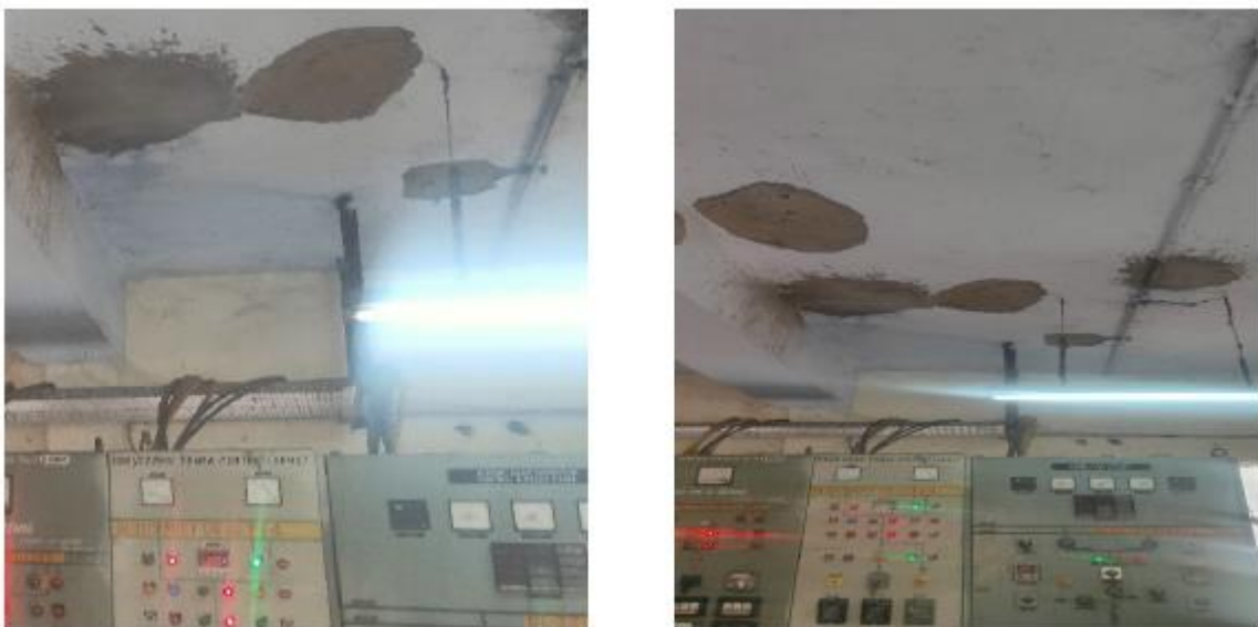
FIG: 12 SHATTERING OF CONCRETE
