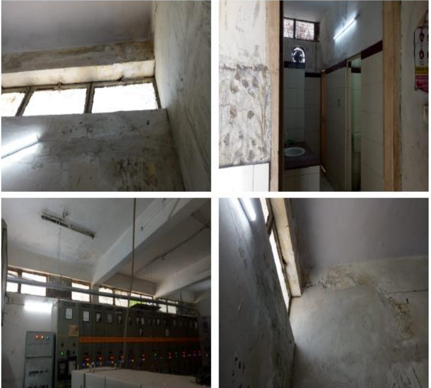
FIG: 8 SHOWING DAMPNESS & SEEPAGE
