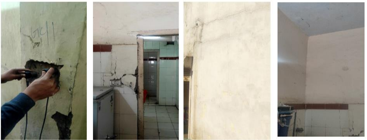
FIG:10 SHOWING CRACKS
